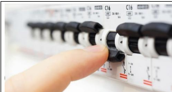
Electric power switched off
